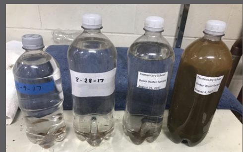
Boiler Loop water samples From right to left: 3 weeks
