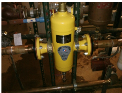
VDT250FA Spirovent – Bldg. 222
